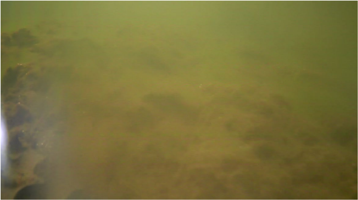
Photograph 5: Underwater still of diffuser pipe covered in sediment and vegetation.
